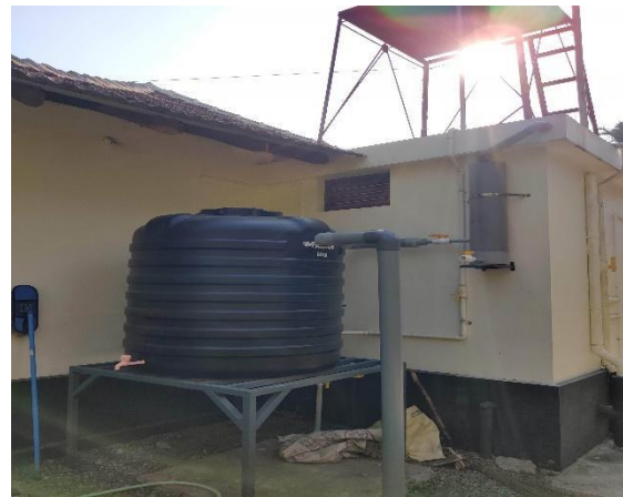
Rain Water Harvesting tanks built in AMRUT
