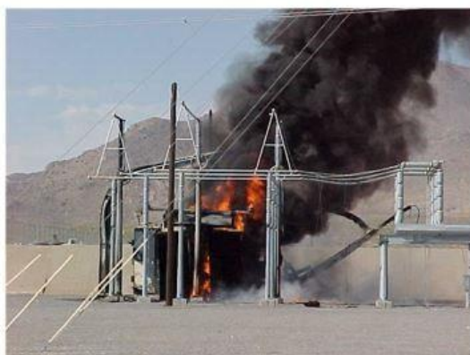
A fire happened in transformer due to electrical fault
